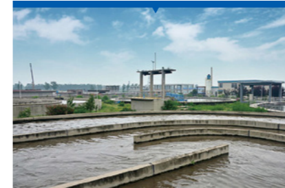
污水处理业 Sewage Treatment Industry
