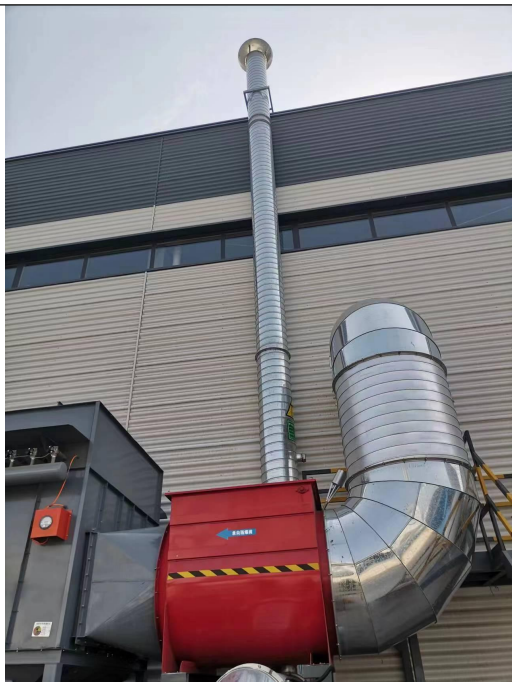
喷漆房排气筒 P7
