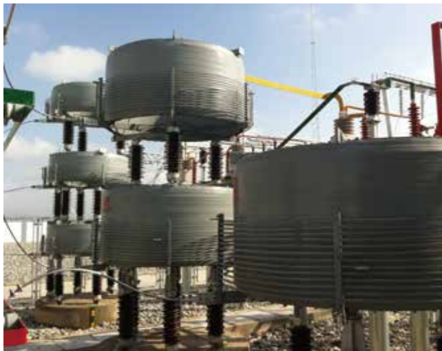
35kV FILTER REACTOR AT A STEEL PLANT (CHINA)
