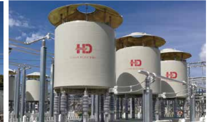
23kV SHUNT REACTOR (SOUTH KOREA KEPCO)
