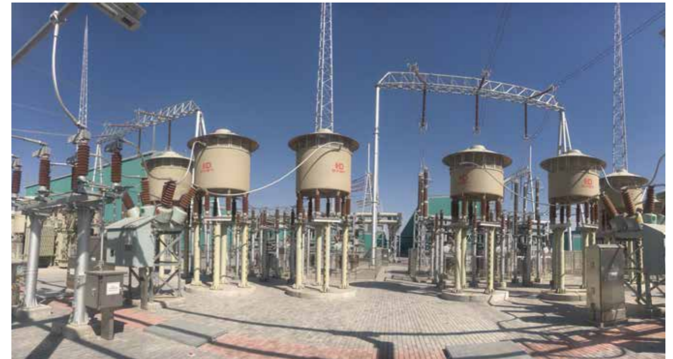
±800kV UHVDC CONVERTER STATION (CHINA)
