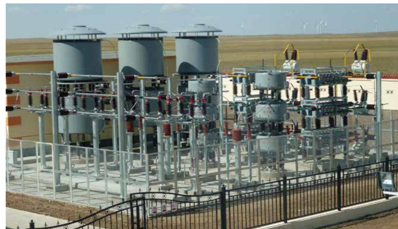
35kV TCR REACTOR AT A WIND POWER PLANT (CHINA)
