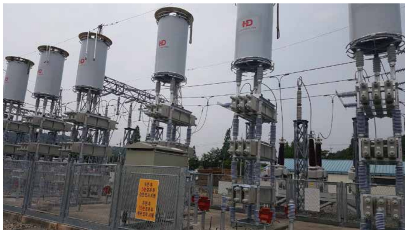
161kV DRY-TYPE AIR-CORE DAMPING REACTOR (KEPCO)
