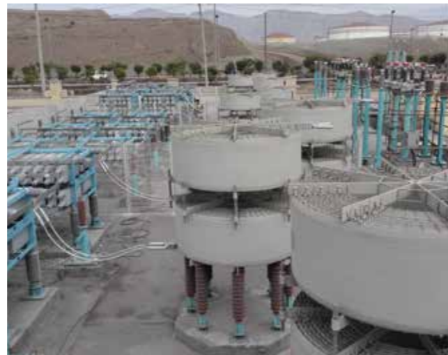
35kV FILTER REACTOR AT A STEEL PLANT (INDIA)
