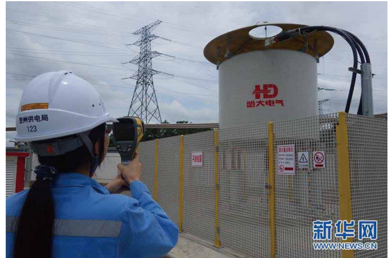
35 kV SMOOTHING REACTOR (CHINA SOUTHERN GRID)
