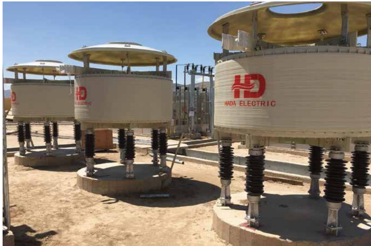
35 kV CURRENT LIMITING REACTOR (CHINA)
