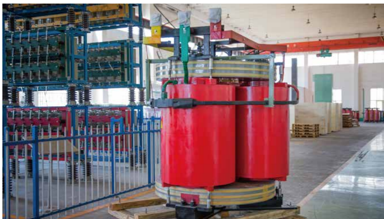
10kV DRY-TYPE IRON-CORE SHUNT REACTOR (CHINA)
