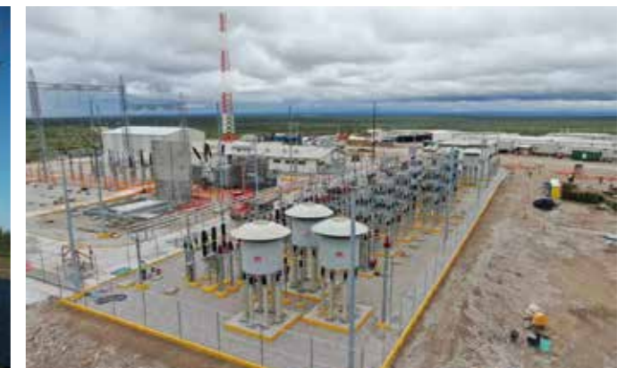
35kV SHUNT REACTOR (MEXICO)
