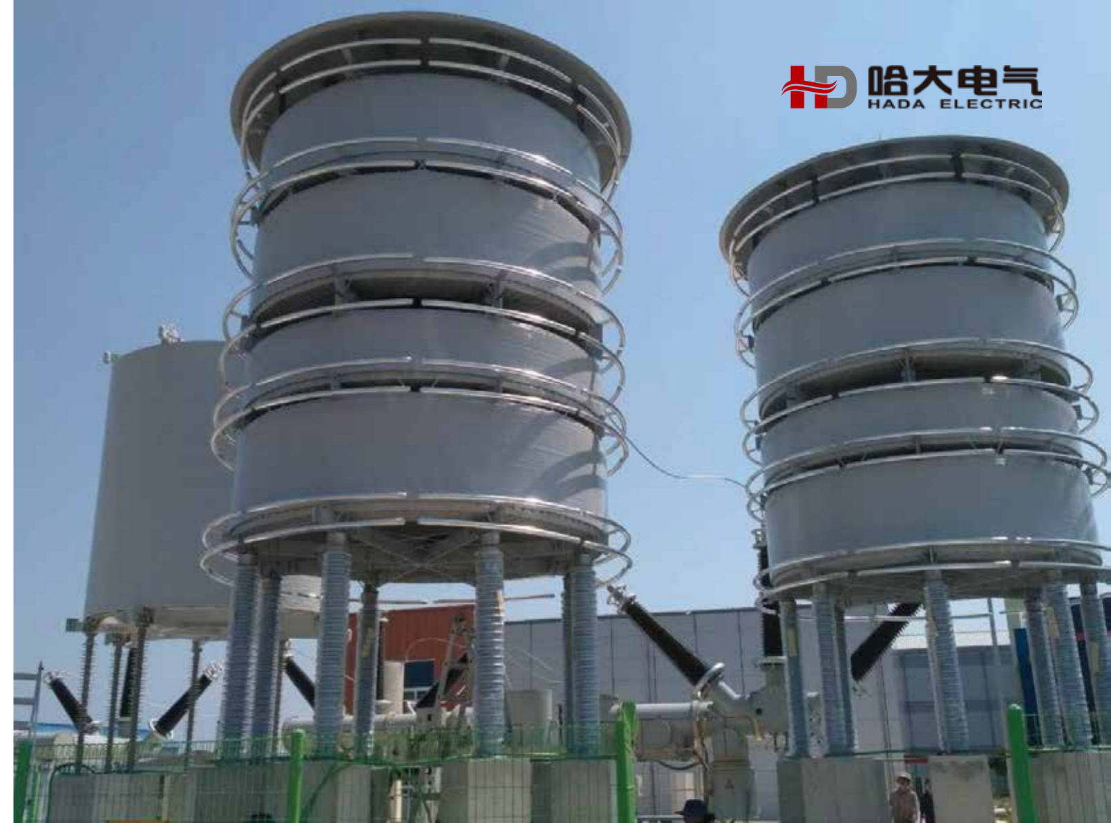
154kV TEST REACTOR WITH TAPS (KEPCO)
