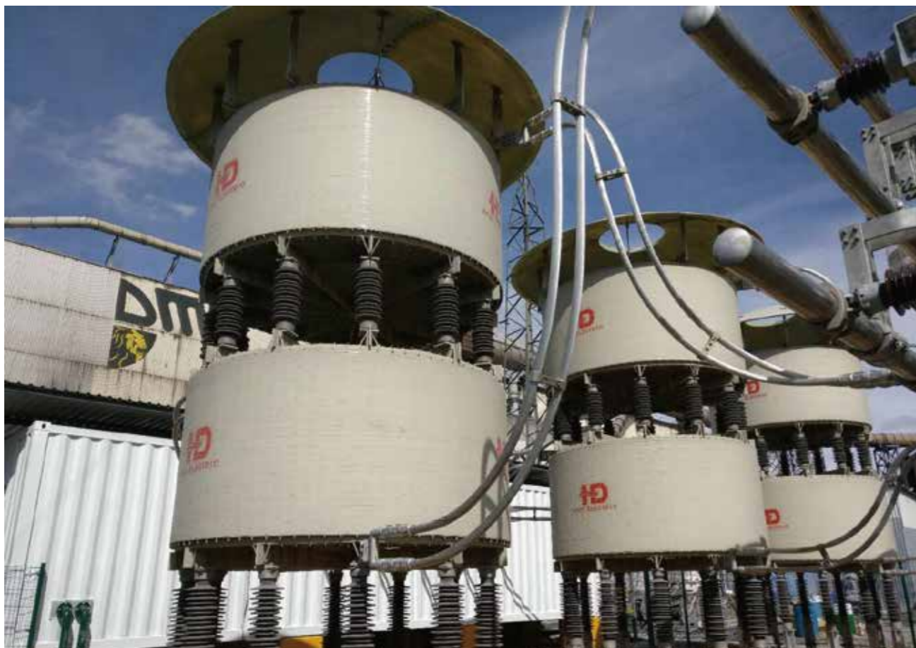
TCR REACTOR WITH RATED CURRENT 2870A (MEXICO ACEROS)
