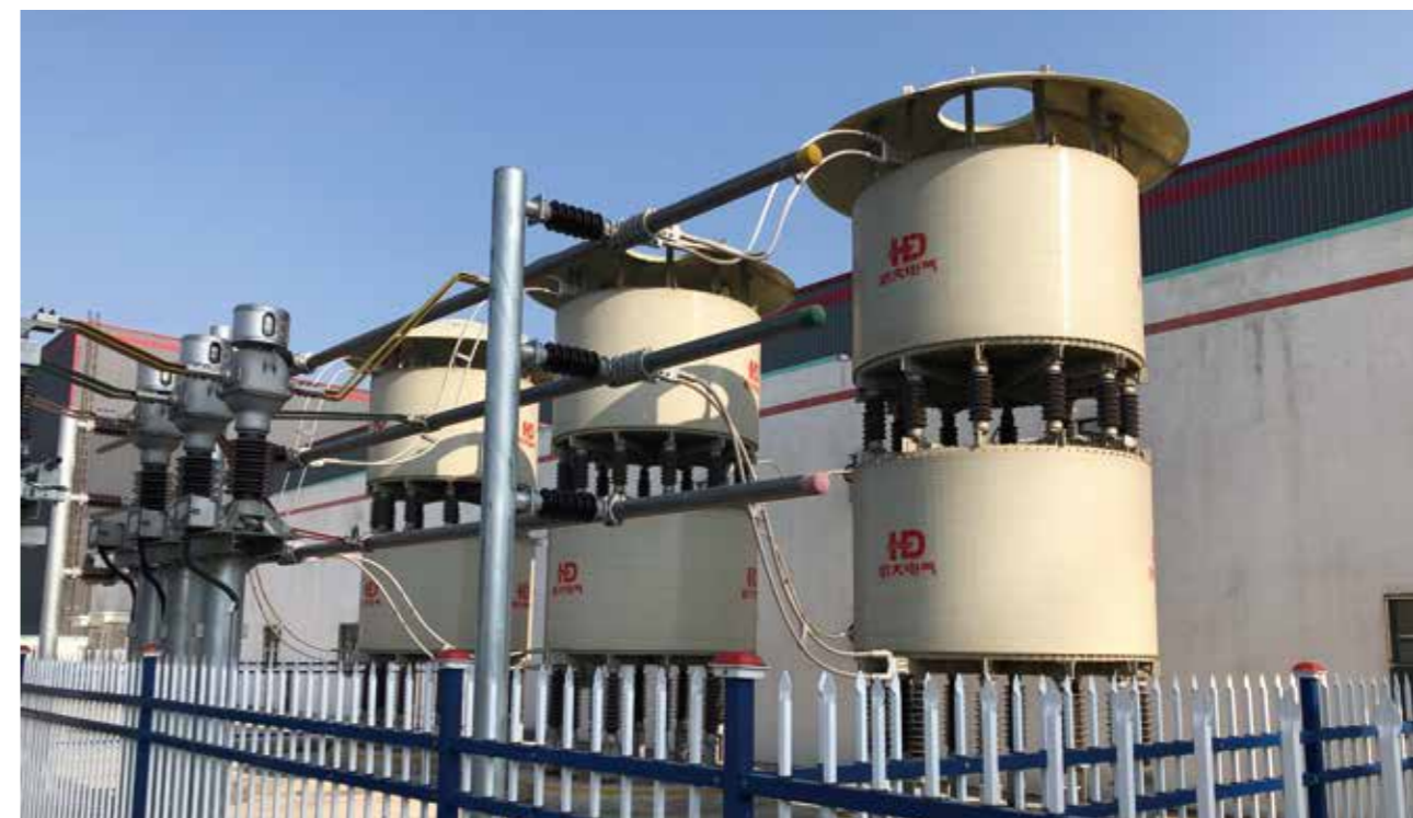
35kV TCR REACTOR AT A STEEL PLANT (CHINA)
