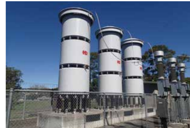
66kV SHUNT REACTOR (AUSTRALIA)
