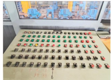
Automation Control Room
