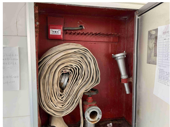
Fire fighting facilities.JPG
