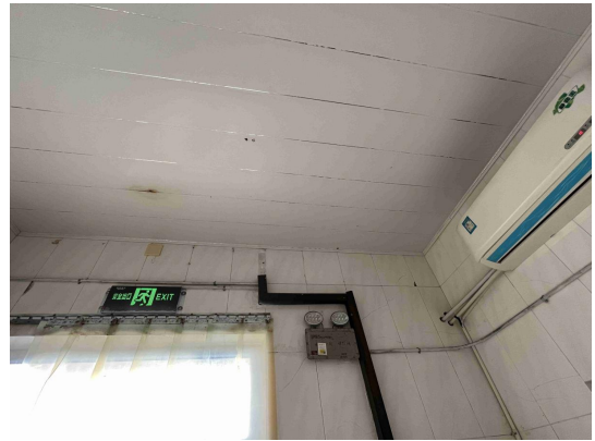
Emergency light and Exit sign.JPG
